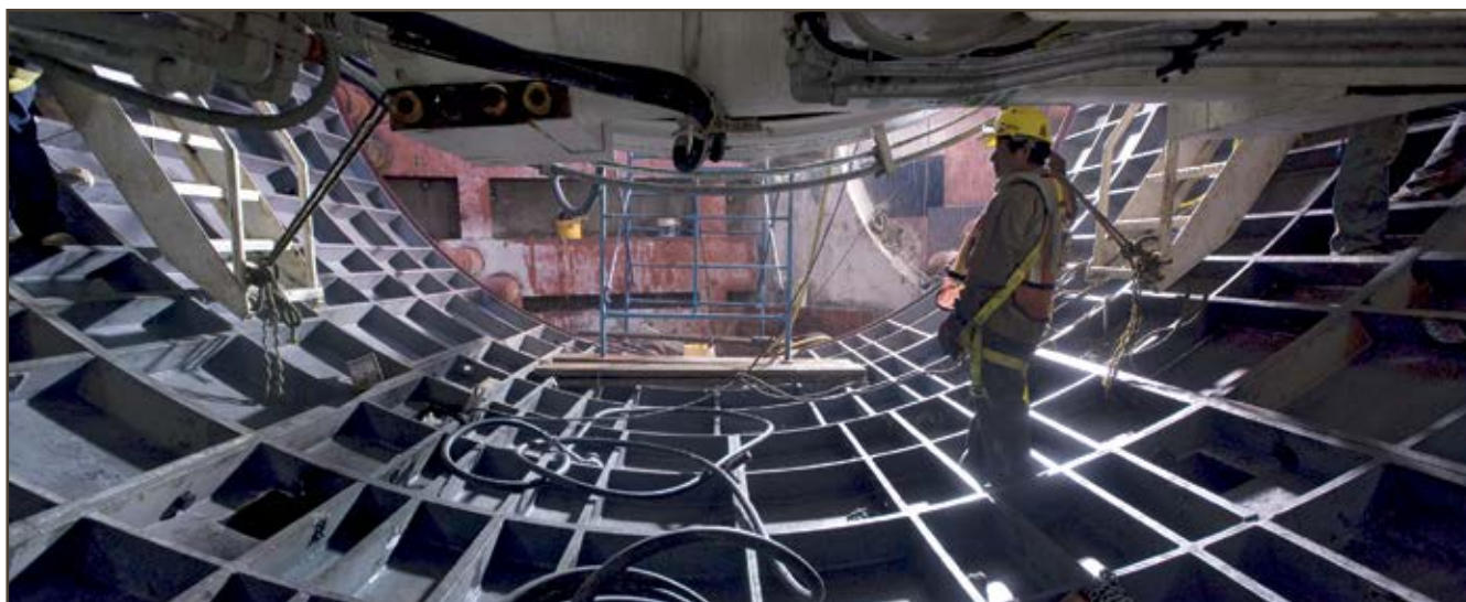
A hydraulics specialist working in the construction of Mexico City's deep drainage system, known as Tunel Emisor Oriente (TEO)
