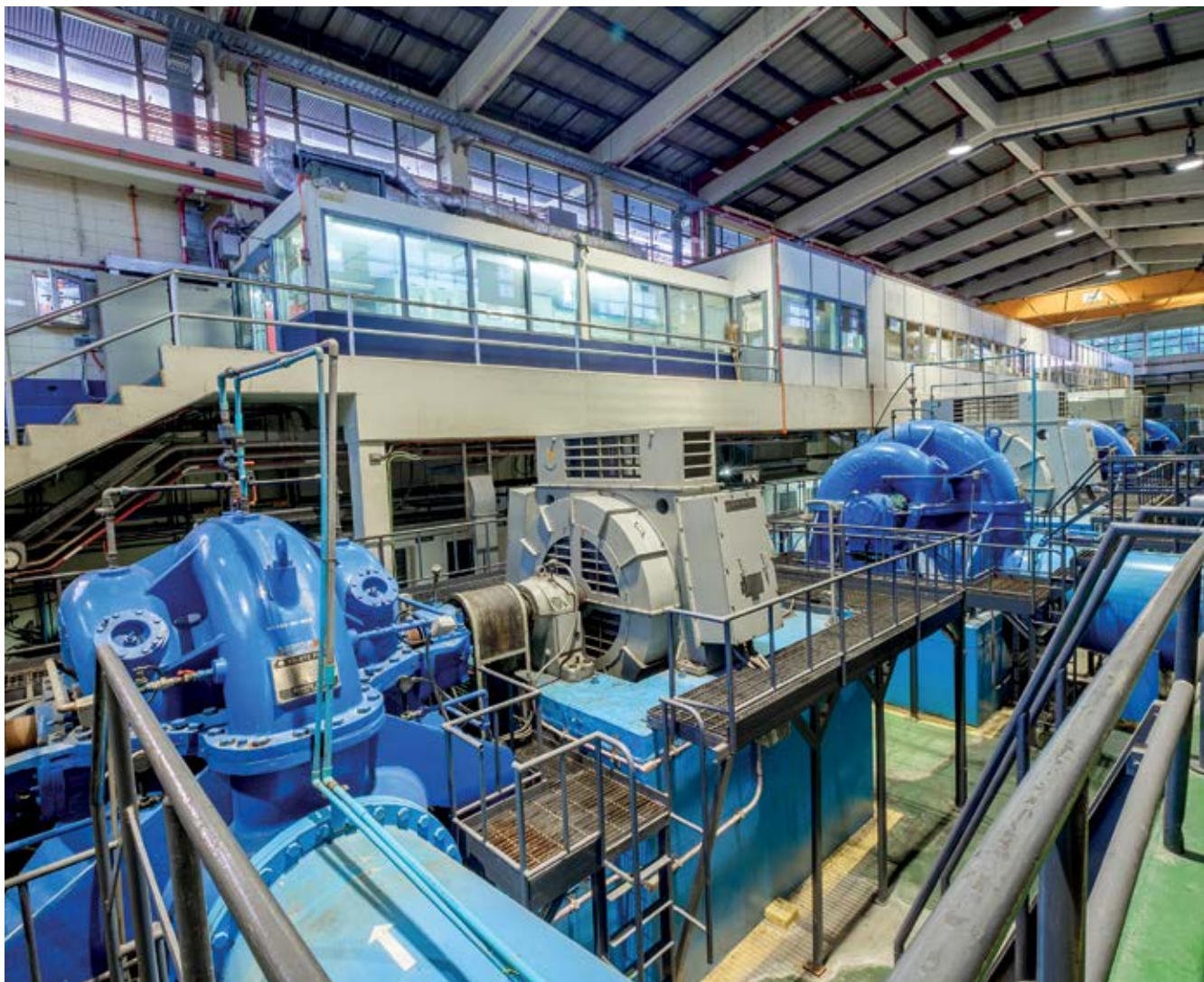
Pumps and motors for pumping water supply in a water treatment plant in Bangkhen, Bangkok, Thailand.
