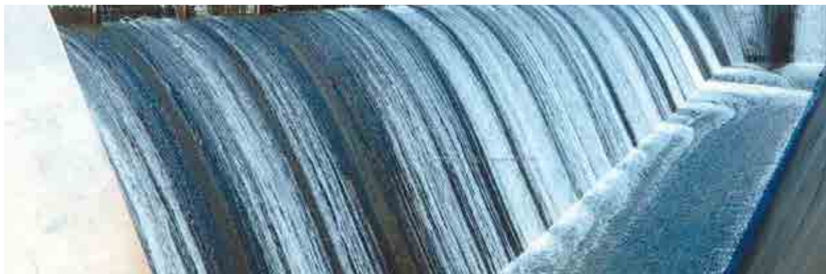
Photograph of barrier showing the overflow spillway of the dam in operation. Ixtlahuaca and Almoloja de Juarez, Mexico, José Antonio Alzate Dam, 1970
